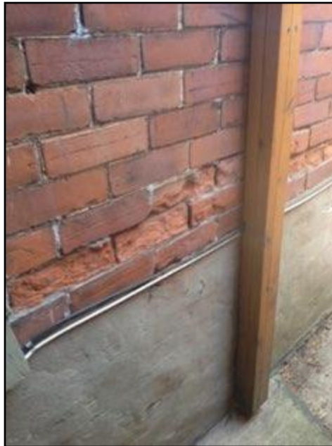
3. Parging damaged or missing
