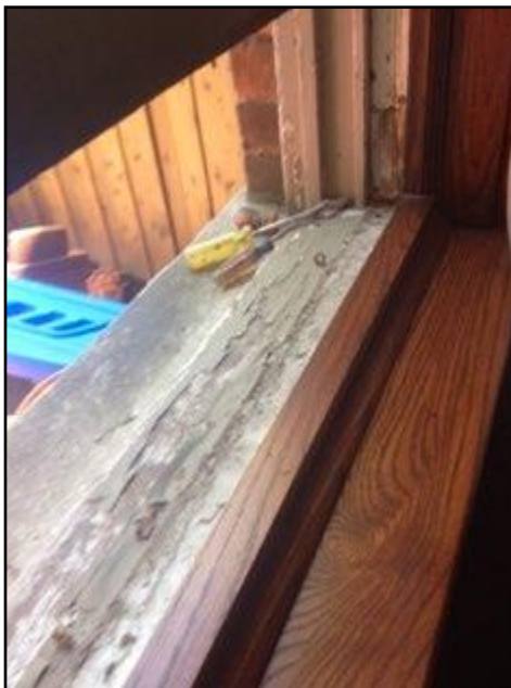
5. Paint or stain needed
