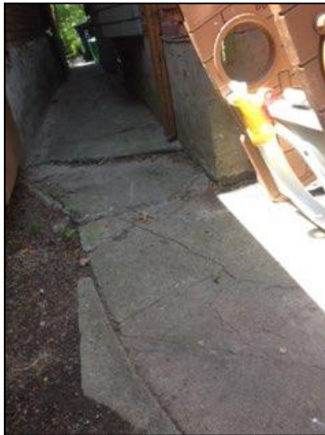
7. Improper slope or drainage
